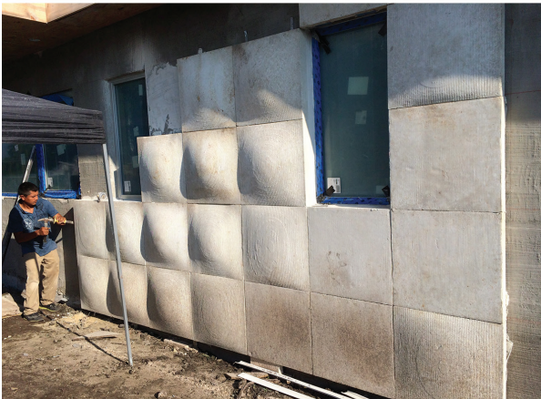
Installation photos of precast wall tiles being hung on existing concrete block wall.
